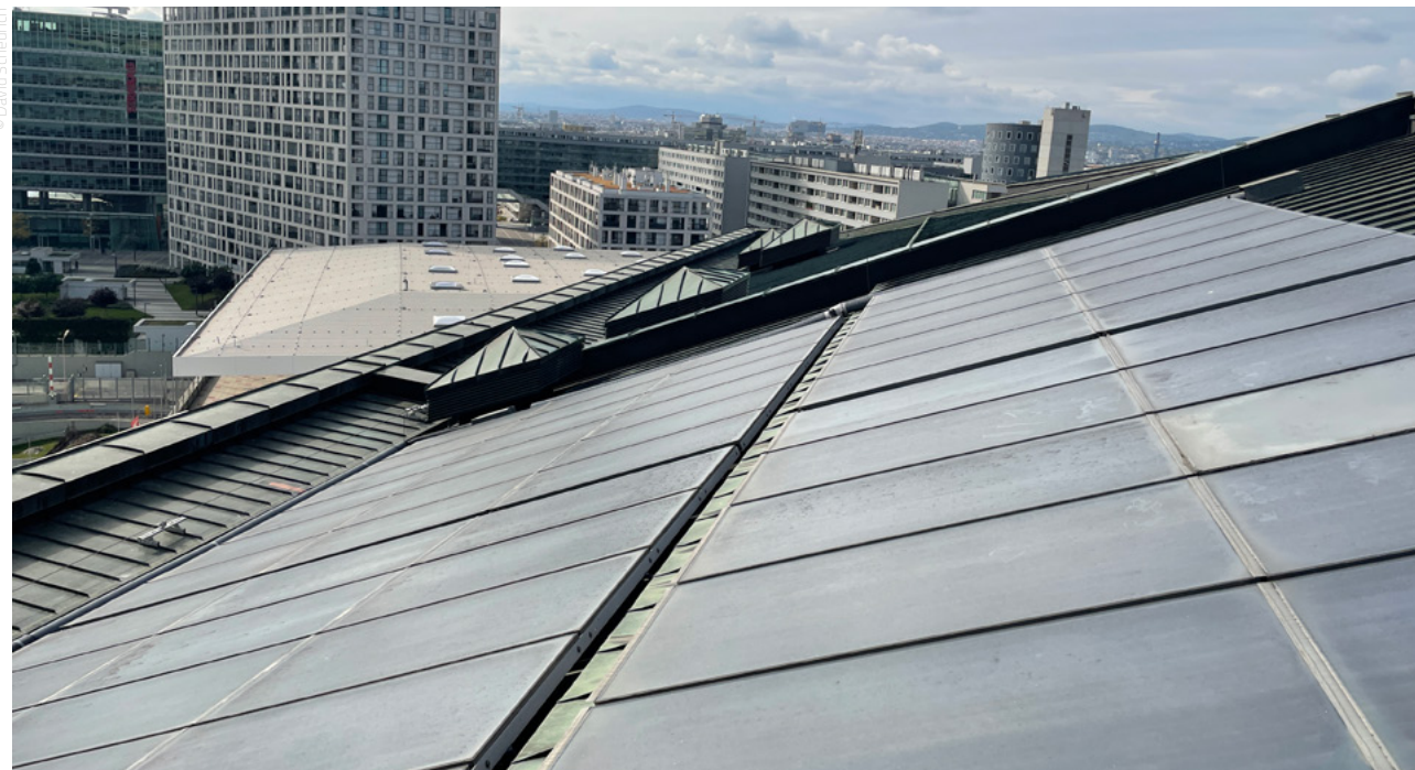
The rooftop solar thermal array supplies the venue with warm water
